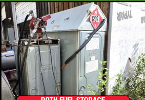
ROTH FUEL STORAGE
