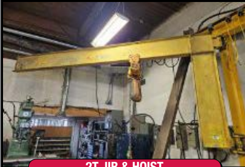
2T JIB & HOIST
